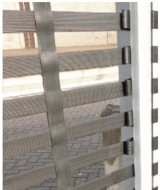
Photograph showing condition of exposed and protected sections of fence (where strips are rolled back - right) after 20 years in service.
