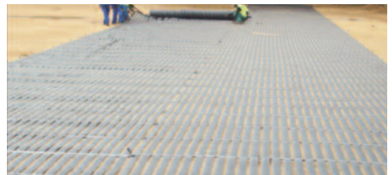
A compacted layer of decomposed granite was placed on top of the geotextile followed by the first layer of GeoGrids of Paralink™ 600 and Paralink™ 1000
