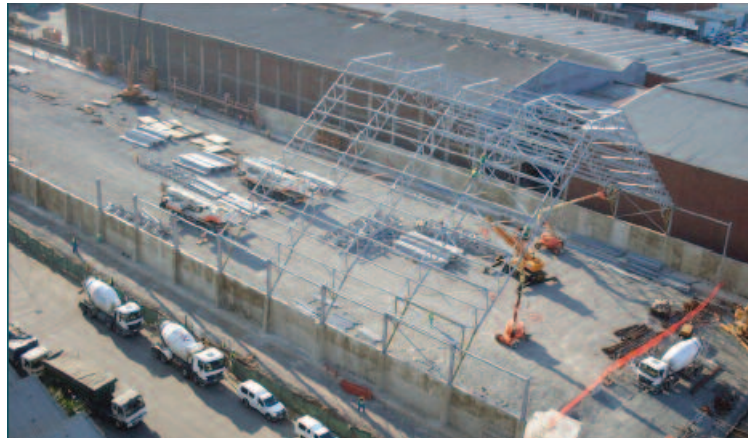
The reinforcing of the approximate 13000sqm foundation of the entire site was completed within six weeks allowing for the structure to be completed within the deadlines set by the shipping requirements.
