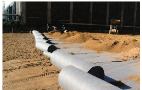
A Layer of the river sand sandwiched between two layers of AG 400 geotextile provided a drainage and separation layer below the proposed soil reinforced raft.
