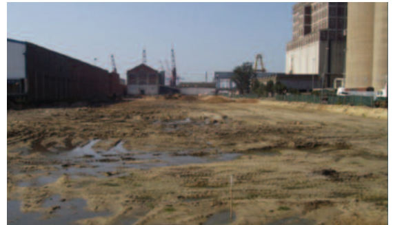
The top 1.5m of in situ material was removed in readiness of the contraction of a reinforced soil raft.
